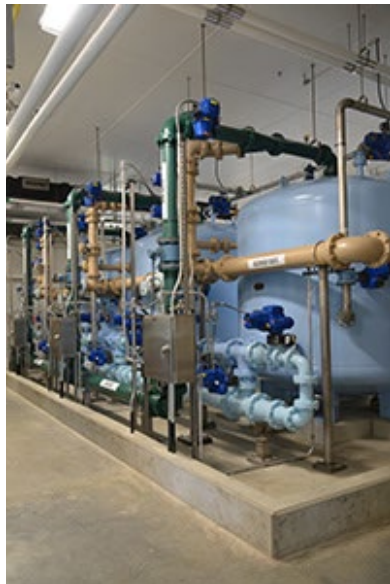
Topsfield water treatment, Source: Public Works
