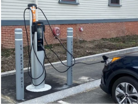
Town Hall Electric Vehicle Charging Stations, Source: Wicked Local 2021.
